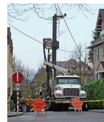
Geo-technical drilling for soil samples helps Sound Transit evaluate soil conditions in a construction area, allowing planners to better estimate resources needed for the project.
